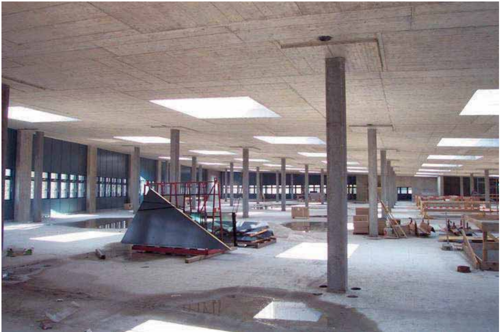
Figure 7 Interior view of the top floor of the empty primary system, showing skylights, openings for light-wells to the floor below (on right of picture), and precast columns with four sleeves at the base of each column for possible vertical drainage piping. Also visible is the inner layer of the double skin envelope, showing operable wooden windows.
