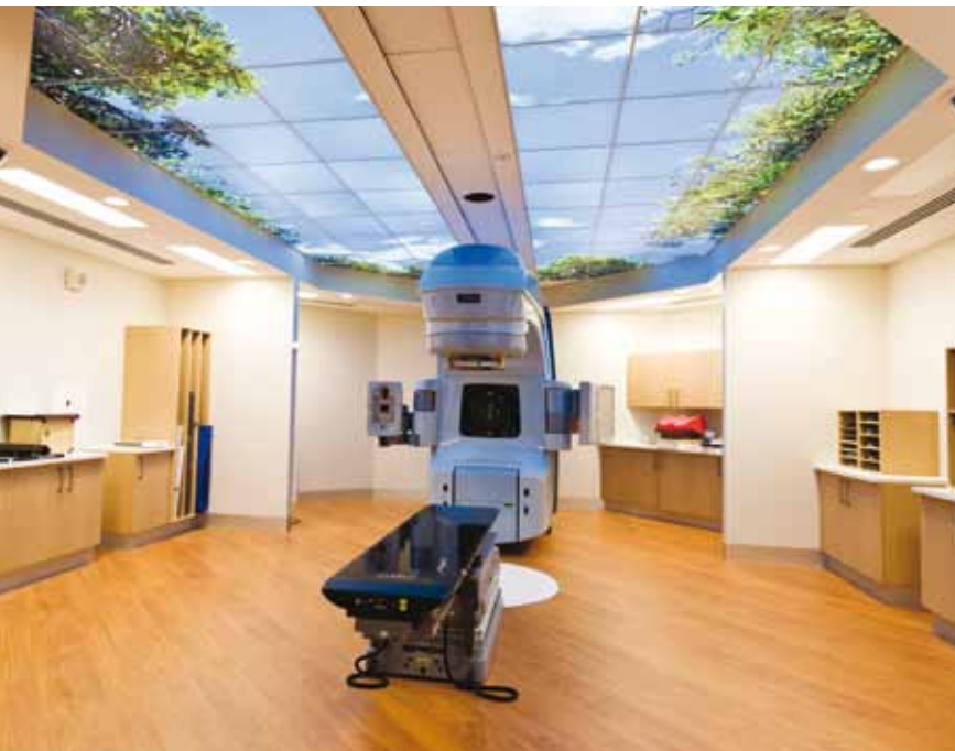
Backlit ceiling panels in the radiation bunkers – one illustrating a tree-top view, another a night sky – act as positive distractions for patients
