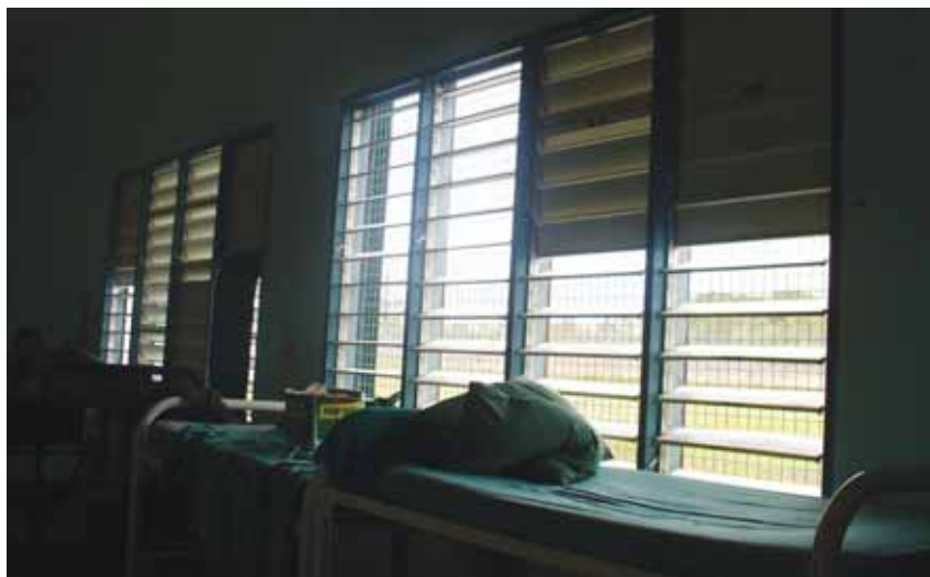
Figure 4: Louvre walls provide cross-ventilation for prisoners' dormitories in the Darwin Correctional Centre, Northern Territory. Darwin is a tropical climate with wet and dry seasons, and rain on occasion enters the accommodation due to the design. No air-conditioned prisoner accommodation is provided at this facility
