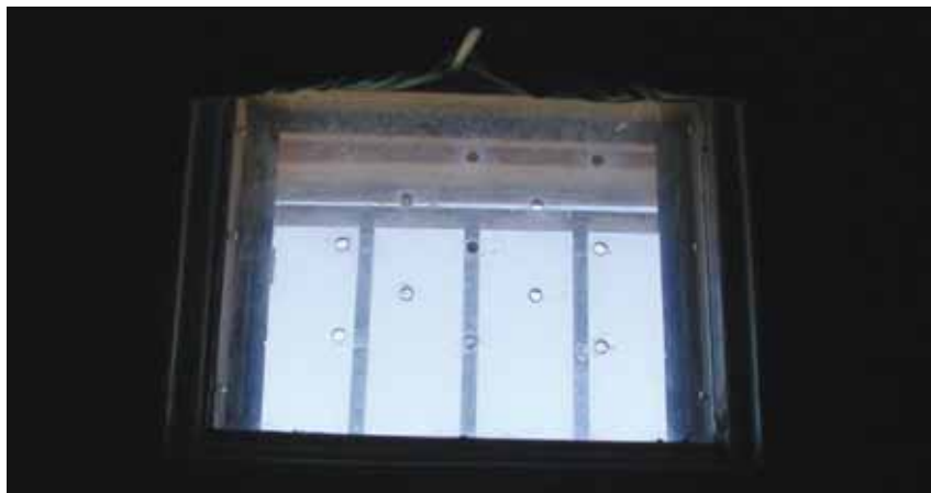
Figure 3: Holes punched in Perspex guards on windows in high-security accommodation at Yatala Labour Prison, South Australia. While the prison is air-conditioned, air movement to the cells is only via gaps under doors, and prisoners are unable to maintain the temperature as rooms cannot be sealed
