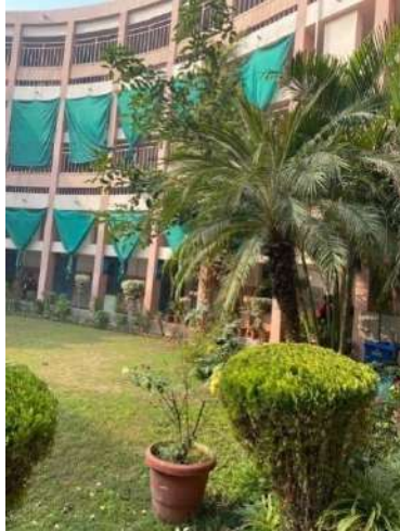
Image 5.23: Poor orientation leading to insufficient ventilation
