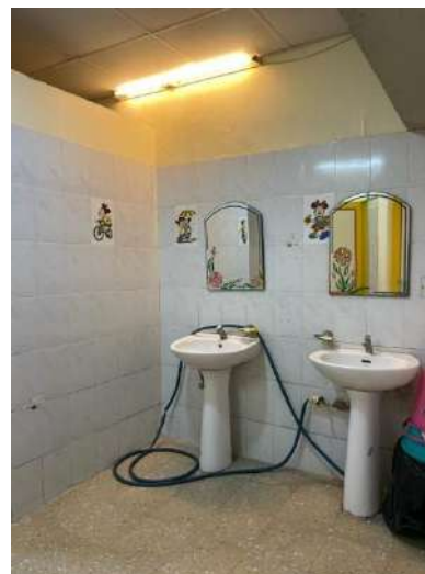
Image 5.6: No height consideration in toilets
