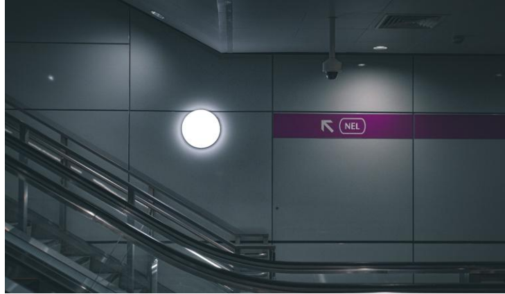
Lights at TEL-NEL Linway in Basement 4 (Outram)
